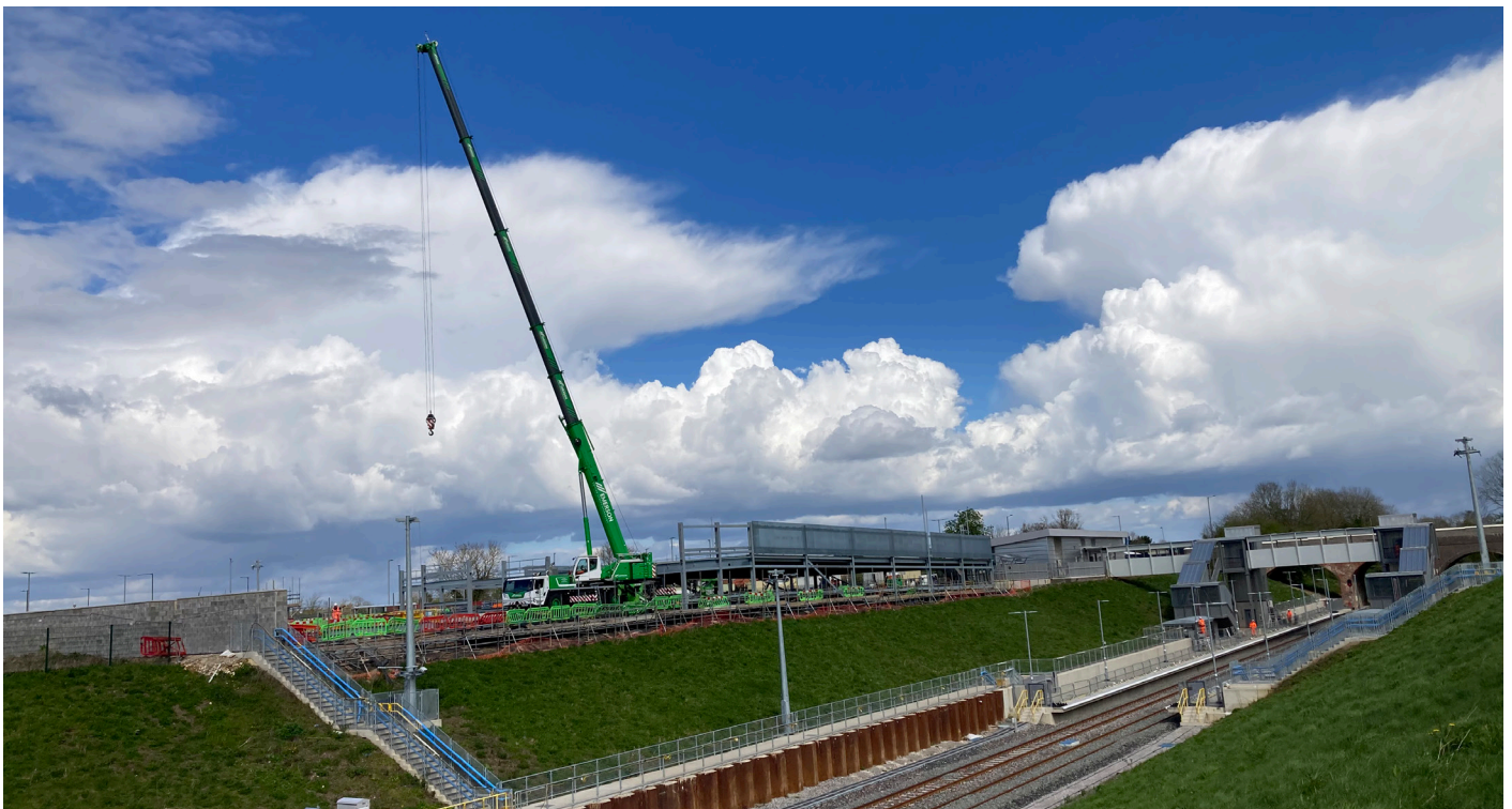
Winslow Station car park construction for Buckinghamshire Council in progress with a crane being used to lift the steel beams and place concrete panels
