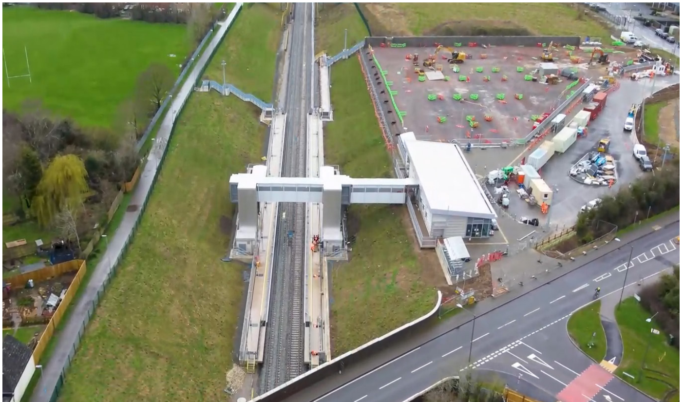
Aerial image of Winslow Station and progress on the station car park, March 2024
