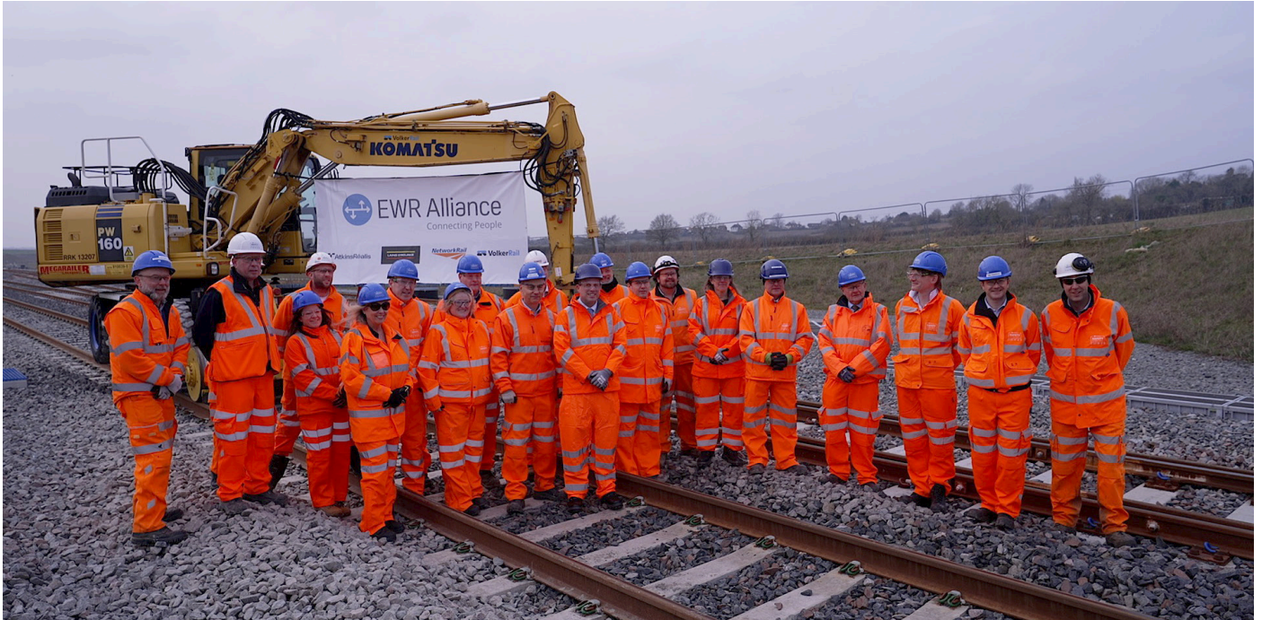
The East West Rail Alliance team with Rail Minister Huw Merriman, Greg Smith Buckinghamshire MP and CEO of EWR Company Beth West marking the completion of track construction from Bicester to Bletchley, March 2024
