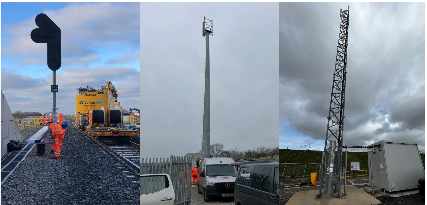
L-R: A signal installed on site, a tower and a lattice tower Global System for Mobile Communications-Railway mast.
